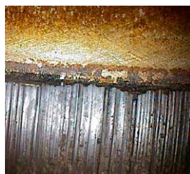
Figure 1 A defected anti-polishing area on liner
